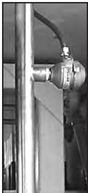
Pictured at the left is a SFI installed in a plant that manufactures ink for desktop printers and copy machines. 100-pound batches of carbon black come out of a feeder and are pneumatically conveyed through a four-inch vertical line. The SFI is used to indicate when a batch of carbon black has cleared the line.
